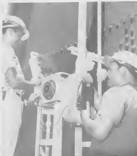
NEWLY INSTALLED automatic tank gauge transmitter is tested for faulty wiring by F. Bikker, left, instrument mechanic A, and his helper R. de Mey. IN AUTOMATIC tank gauge installed recientemente a worde acheck pa waya defeto door di F. Bikker, robez, y su helper B. de Mey.
